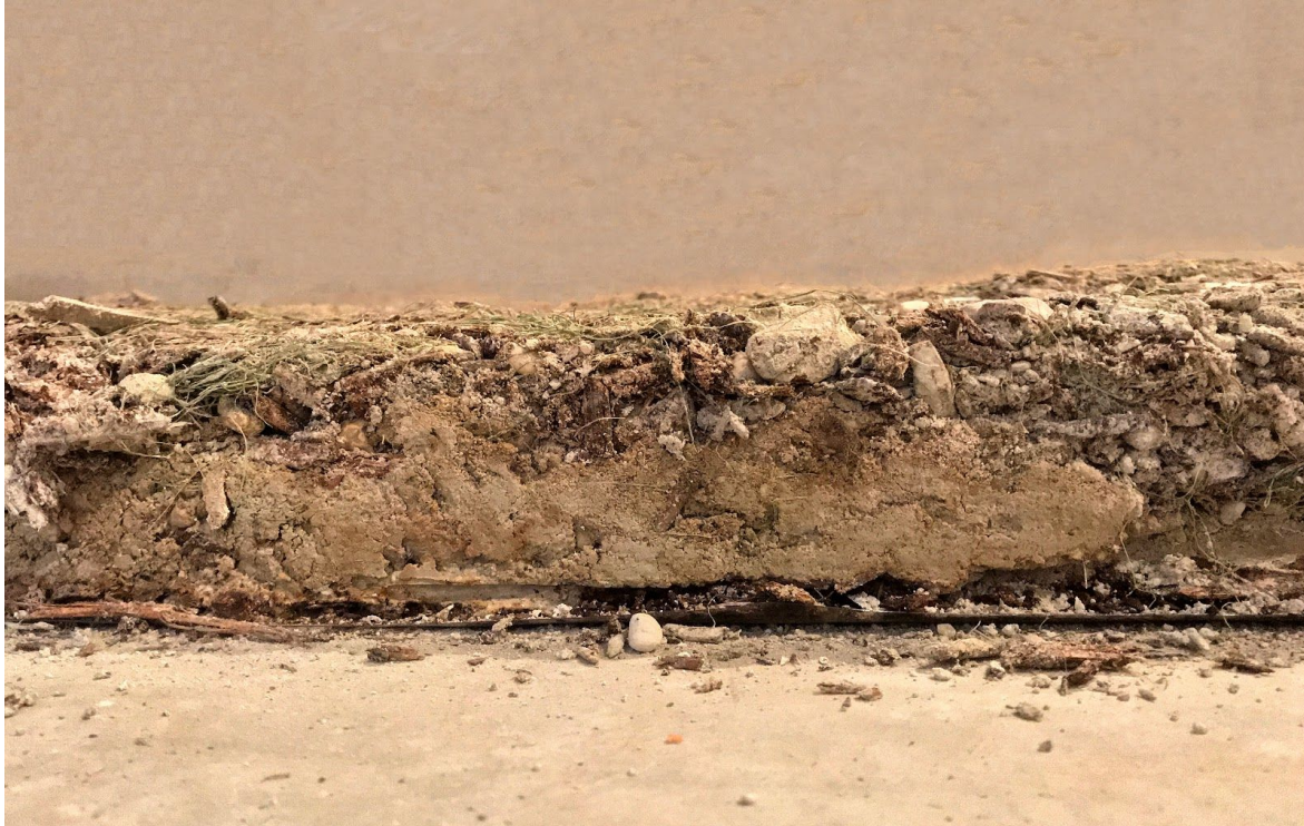
(Figure 3, taken in the bad Barn lighting) One week post concrete, side view.
