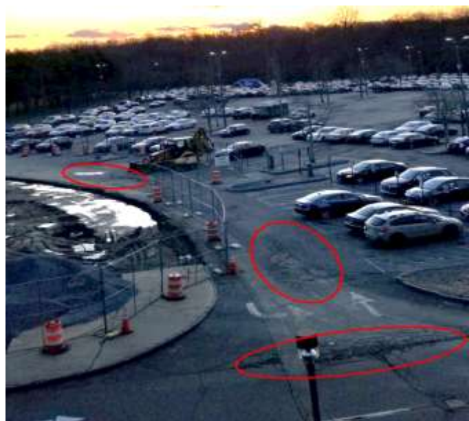
Figure 17 A view of West 2 from the music building with red circles around examples of damage (February 2020).
